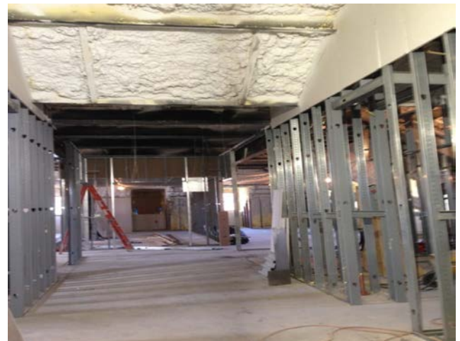
Fernow Hall Third Floor – Wall framing to create future Graduate Student Offices.
